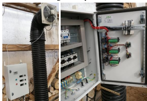
Fig. 3. Greenhouse heating and cooling control unit
